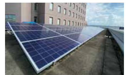
Solar panels on the roof of ALSOK Gunma Head Office
